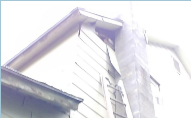
Before: dilapidated siding
