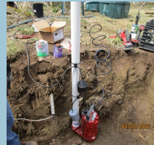
After: New Pump
