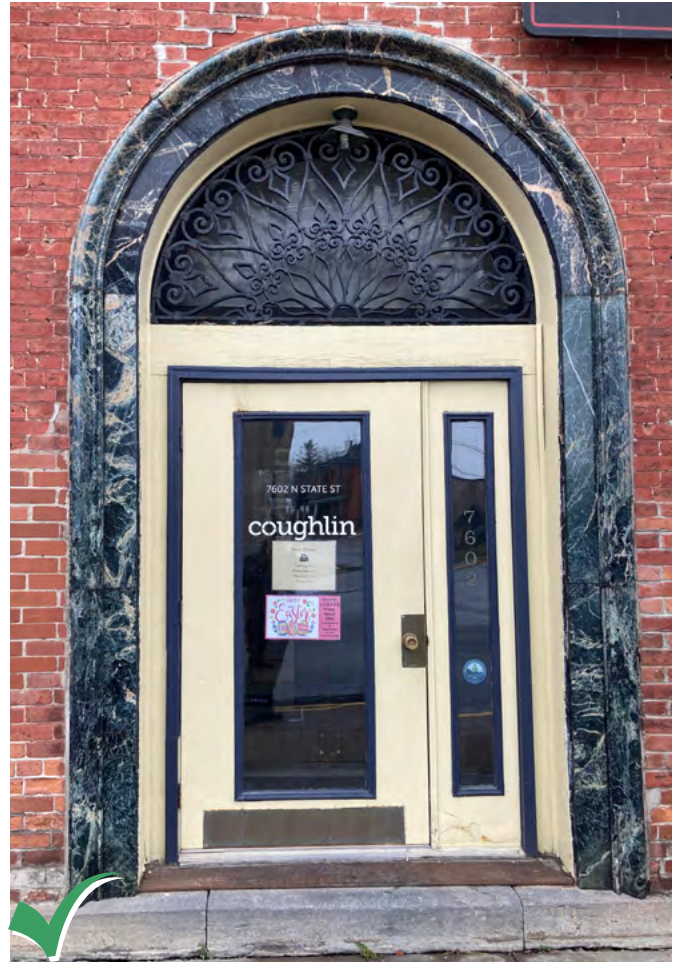
Restore and repair stone and masonry work around side and rear building entries.
