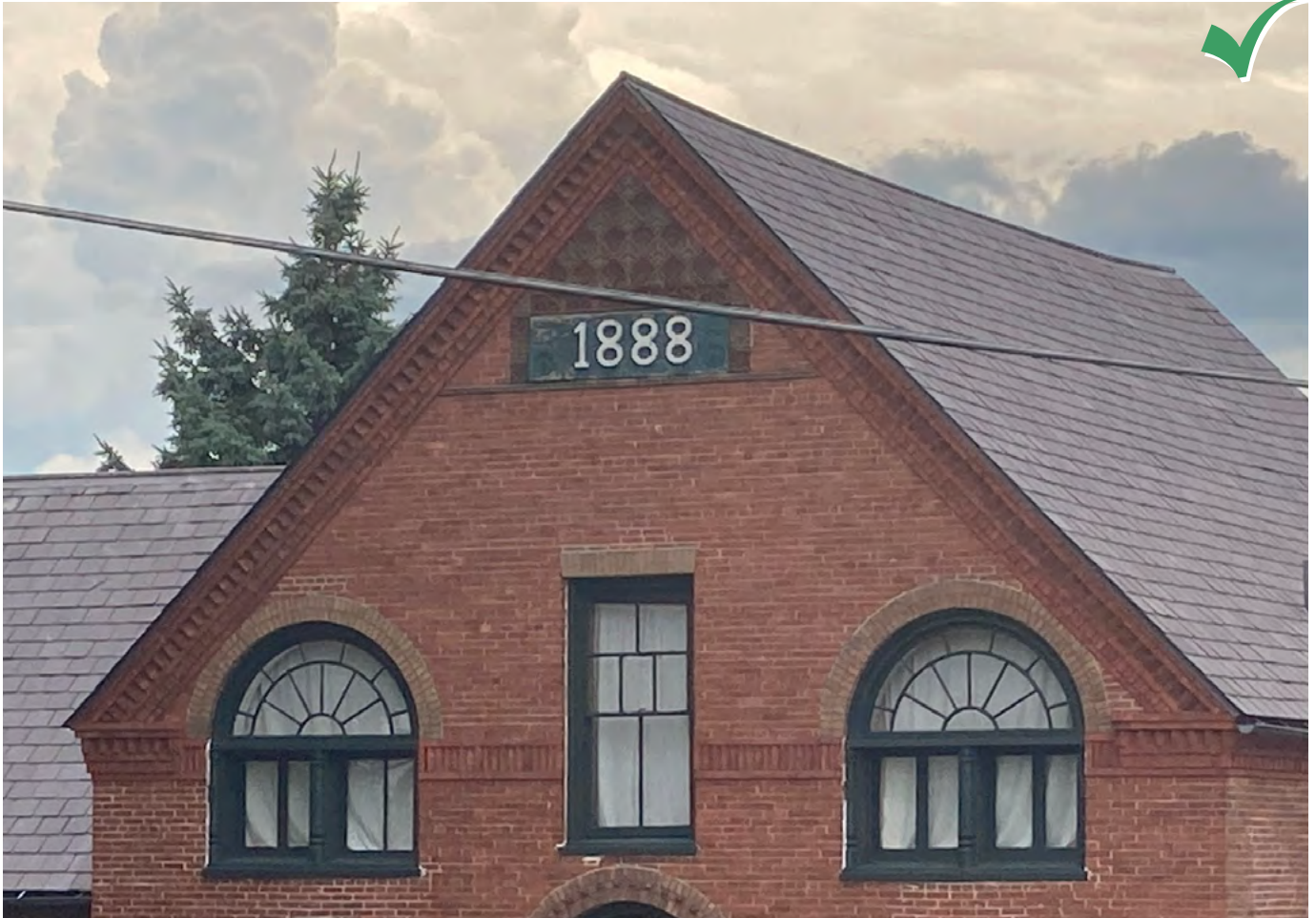
Restore and maintain historic leaded glass transom windows, cornices, and masonry detailing when possible.
