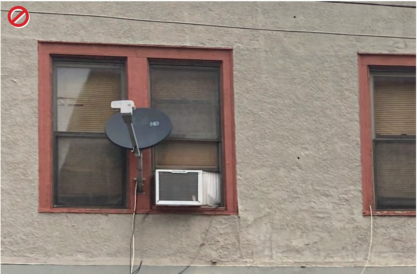
Eliminate clutter from main street facing windows to avoid safety issues and provide a neat and tidy building frontage.
