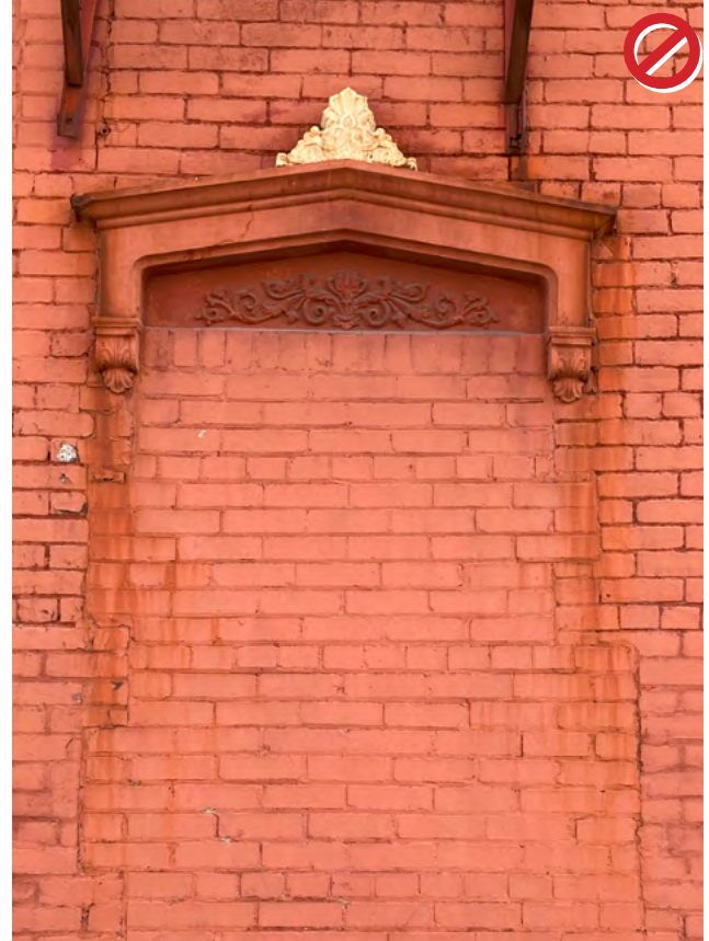
Remember; rust and material degradation stain adjacent materials over time.
