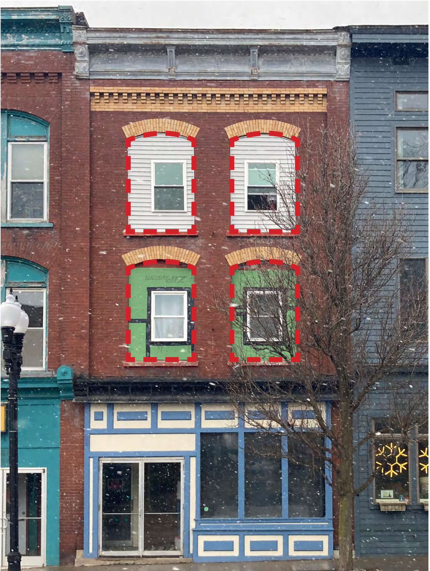
Replace upper floor windows with full size replacements. Do not utilize non-original materials to infill the area around undersized windows.
