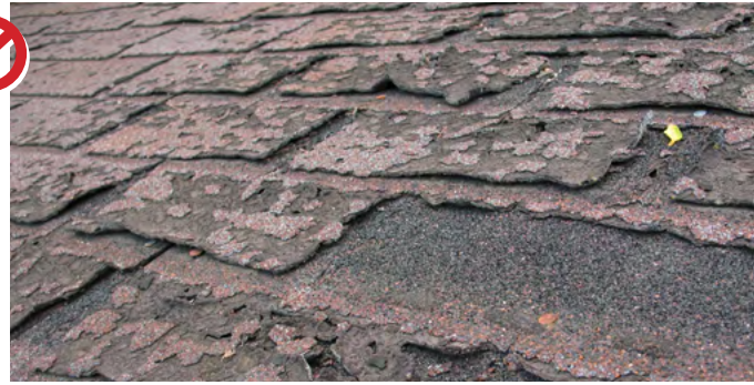
Replace asphalt shingles that are past their lifespan with a more durable alternative.
